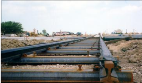
Embedded track construction with new continuous welded rail wrapped in the Ironhorse “Boot”®, fastened to steel ties.
