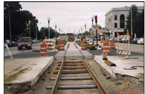
By using steel ties where track runs through pavement, the cost of the in-street track was reduced.
